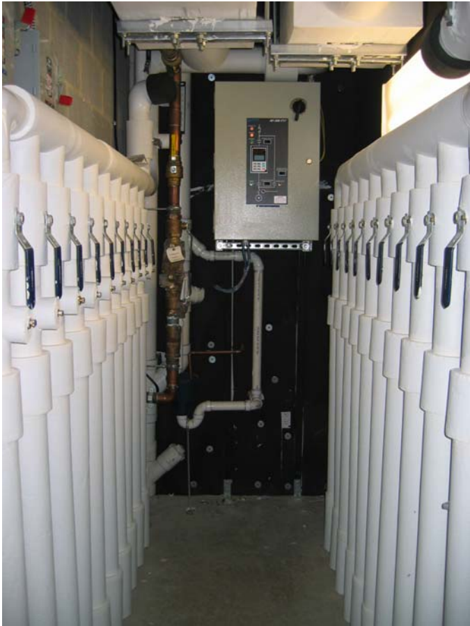
After Installation - Mechanical Room/Heat Pump
