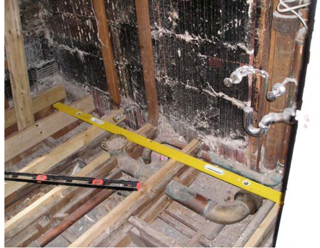
DURING PICTURE – Some re-plumbing was required to correct previous work based on new design.
