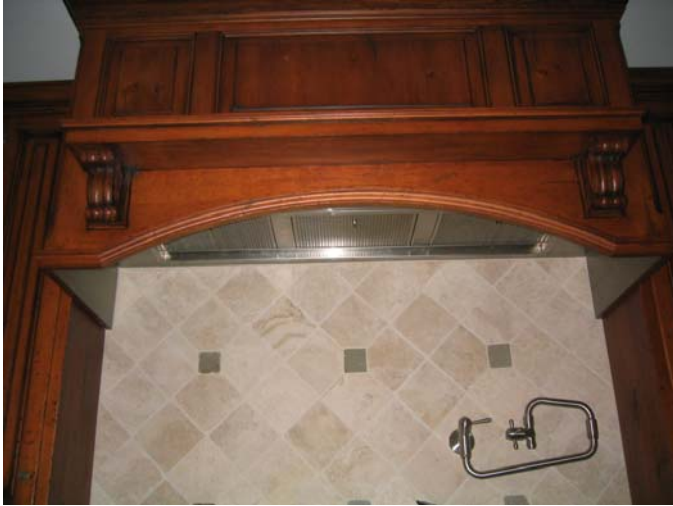
AFTER PICTURE – View Of Exhaust Vent Above Cook Range.
