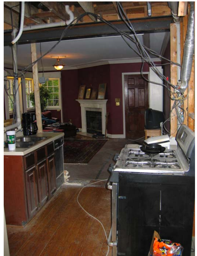
BEFORE PICTURE – View of exposed steel beam, joists & plumbing lines left unfinished by previous contractor.
