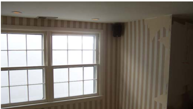
BEFORE PICTURE – View of the window side where the bump out option to increase kitchen room will be applied.
