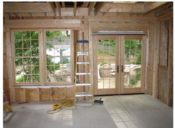
Design proposal called for an open space between kitchen and family room, installing columns was necessary.
